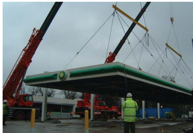
The Global-MSI canopy built for BP, at Gatwick Airport, West Sussex in 2005
