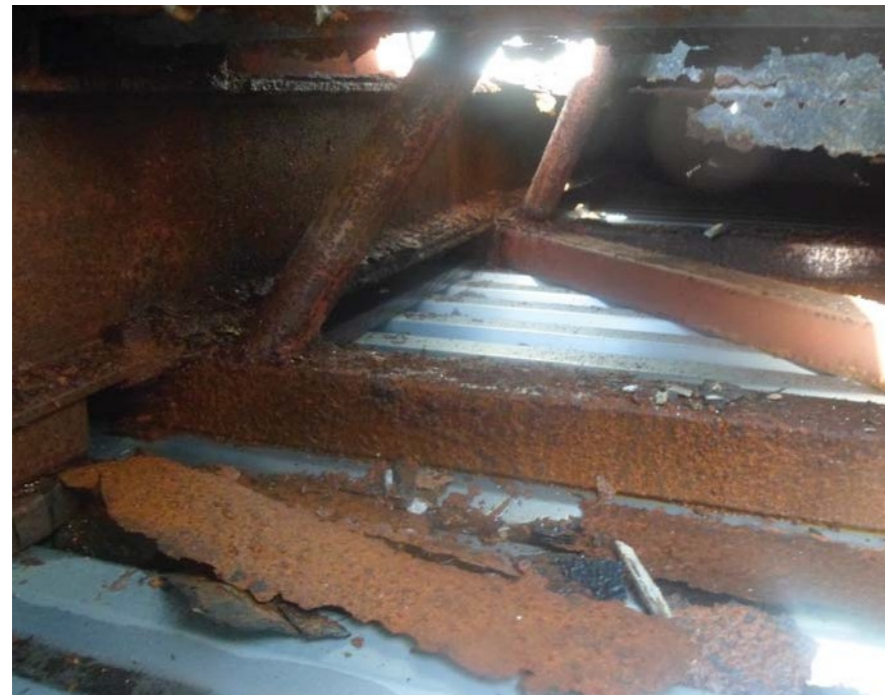
The above photographs show the extent of accelerated corrosion due to air pollution on a series of profiled steel roof sheets. The resulting damage has caused the roof deck to lose watertightness exposing the supporting steelwork below to acidic rainfall and increased moisture
