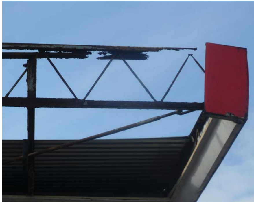
This photograph was taken following the winter storms of 2013/14. During windy conditions, image fascias and sheeting became detached from the canopy. The extensive corrosion of the canopy steelwork was a major contributing factor."
