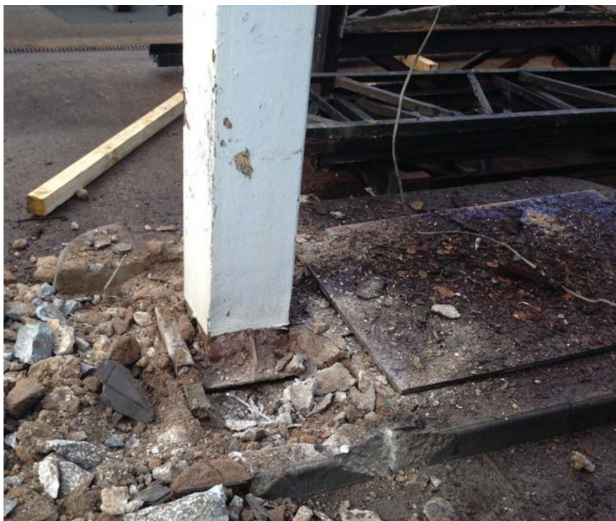
These two photographs were taken during the dismantling of a filling station canopy in February 2014. Global-MSI's concerns are not just limited to poor condition and lack of maintenance of canopy roof structures. The canopy columns above have no holding-down bolts securing them to foundations. They were simply placed onto the forecourt slab and covered by the pump island.
