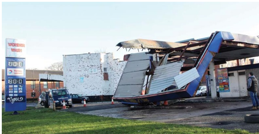
The above photograph shows a former filling station canopy at a car wash premises in Greater Manchester following collapse in February 2014 (the 'A-frame' is still visible protruding above the collapsed structure). The external appearance of the canopy would have given little indication of the endemic deterioration the main canopy deck steel members had suffered. It is cases such as this that strengthen Global-MSI's belief that in the near future an ageing UK filling station canopy will suffer a sudden structural collapse.
