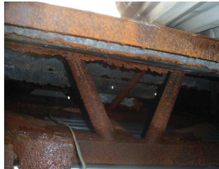
These two photographs were taken during recent surveys of filling station canopies that have exceeded their intended 25 year design life and the indicated damage typifies that of ageing canopies that have not been regularly maintained. The first photograph is from the same canopy supplier as the partially collapsed structure featured above. The second photograph shows a loose bolt forming the connection of two primary structural beams – a common occurrence increasingly being witnessed by Global-MSI's surveyors.
